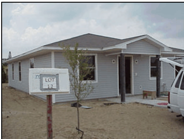
Figure 20. Sealed attic home under construction in Ft. Myers, FL. Conventional dark gray shingles were used.
