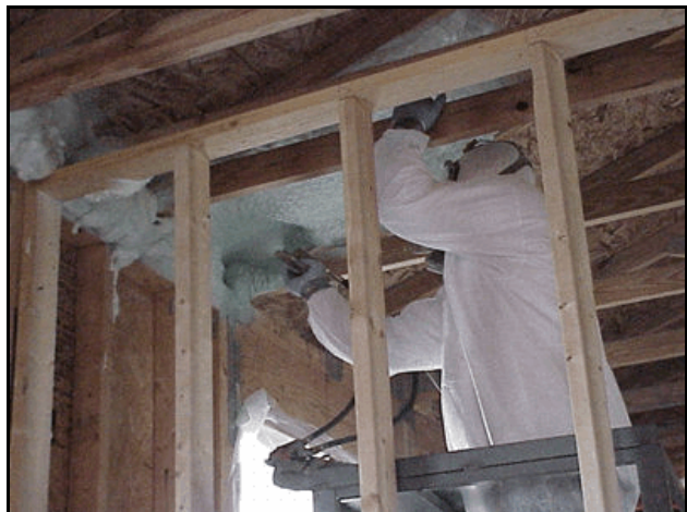
Figure 21. Insulating foam being applied to a 5-inch depth on the under side of the roof.
